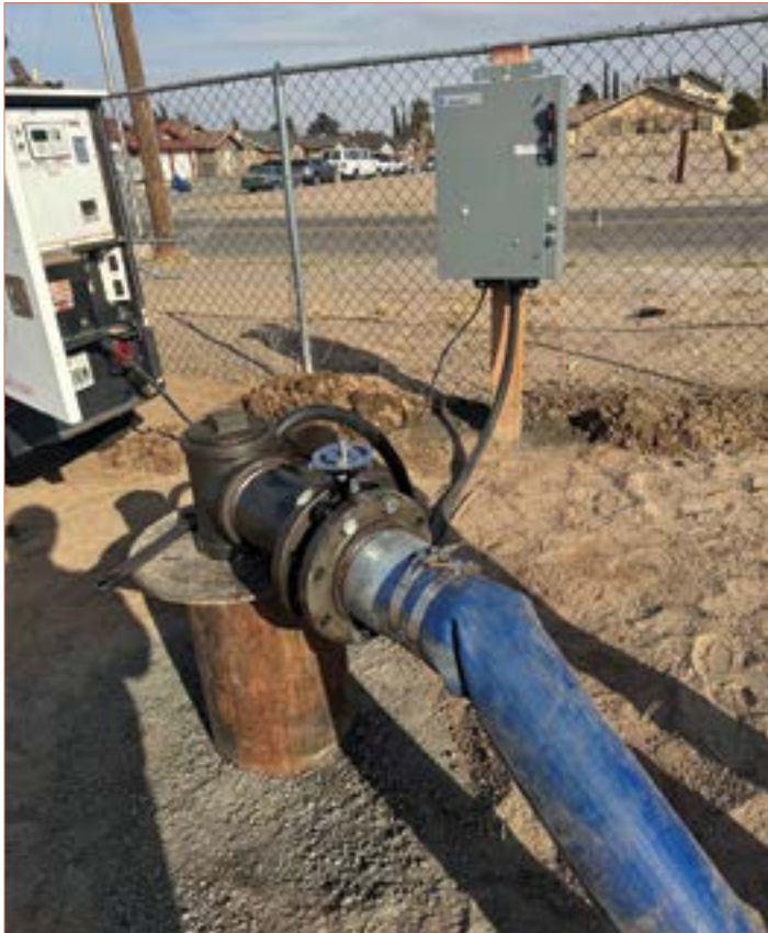
● A newly installed well water pump for the corn field located on Socorro Road that is being used to farm traditional corn. This installation will allow for irrigation of the traditional cornfield that will be used for traditional events.
